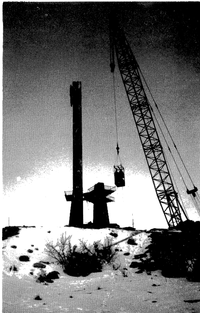
Workers were transported to work platforms to weld adjoining segments of the triune cross tower.
