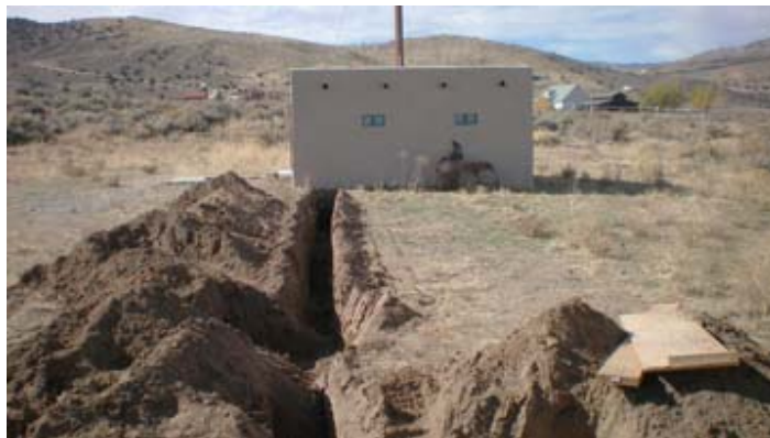
Pump house and trench to first pull box. PHOTO: Ted Staver
