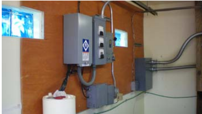
View of some of the inside electrical fittings in the Argonaut pump house. PHOTO: Ted Staver
