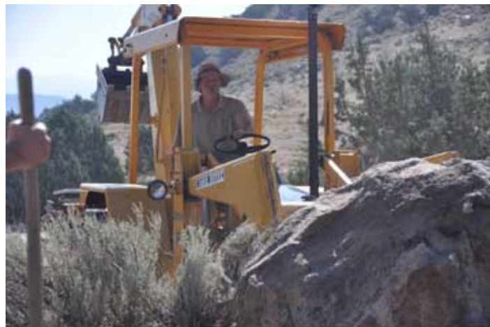
Ted Staver moving earth at the Sanctuary for water lines. Photo: Stephan Fuelling
