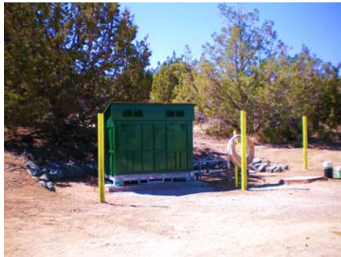
Completely outfitted lift pump station PHOTO: Ted Staver
