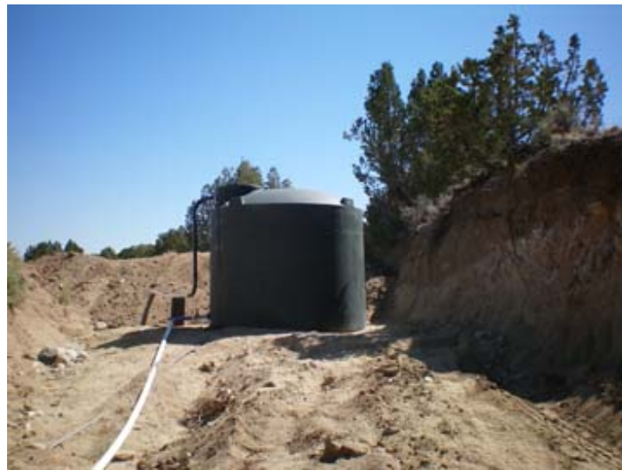
Water tank set up between pond and lift pump station. PHOTO: Ted Staver
