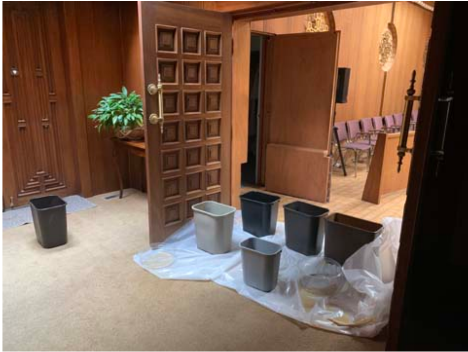
Leaks at Chapel entrance
