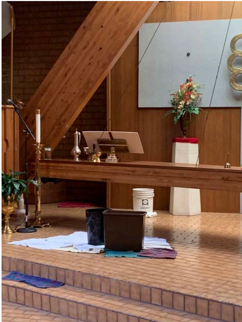
Leaks at Chapel chancel area
