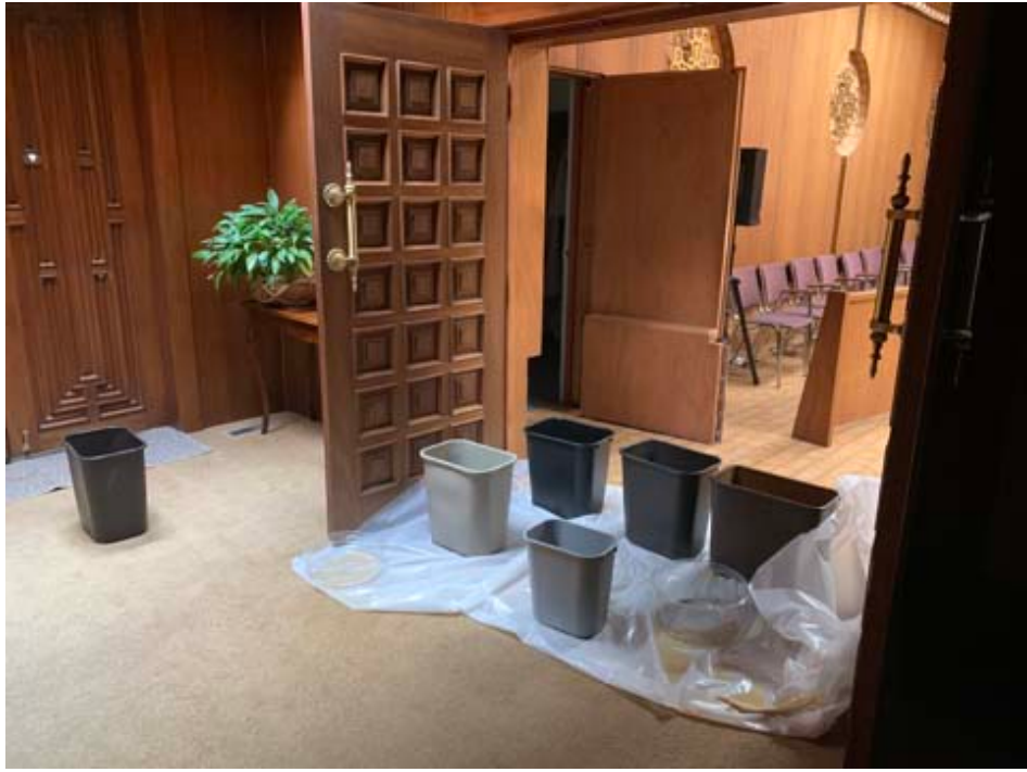
Leaks at Chapel entrance
