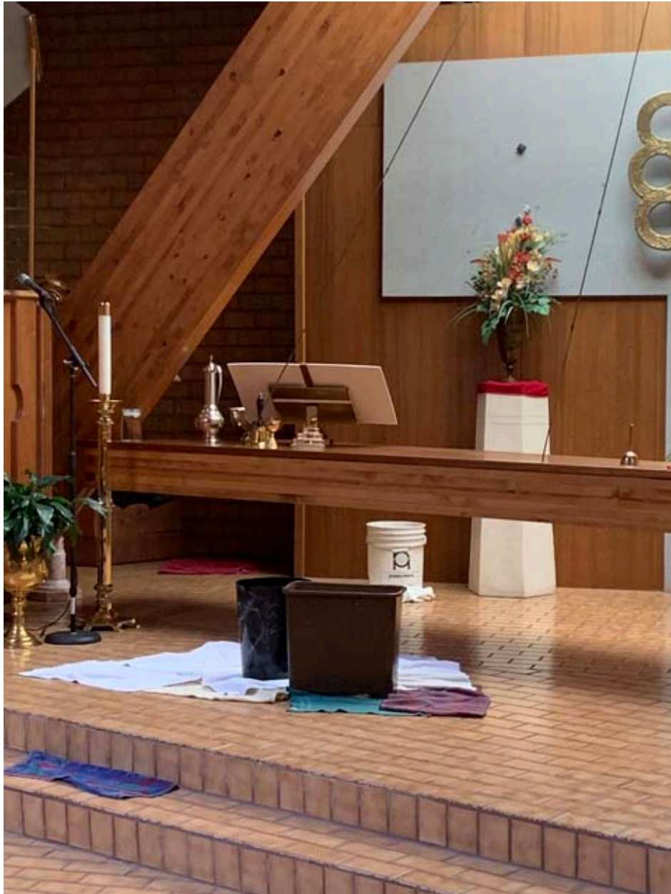
Leaks at Chapel chancel area
