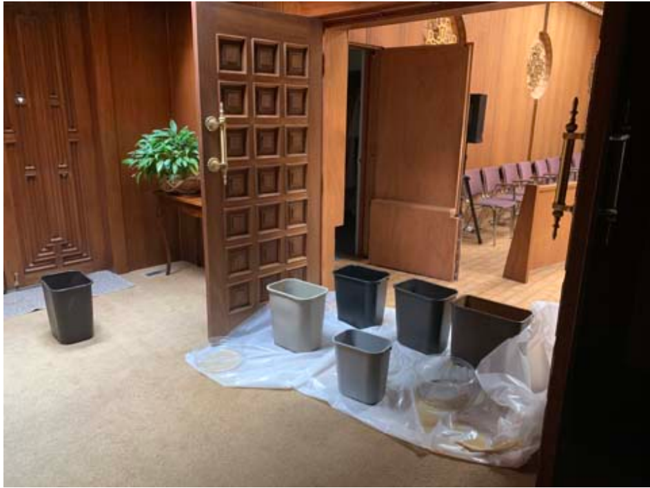
Leaks at Chapel entrance
