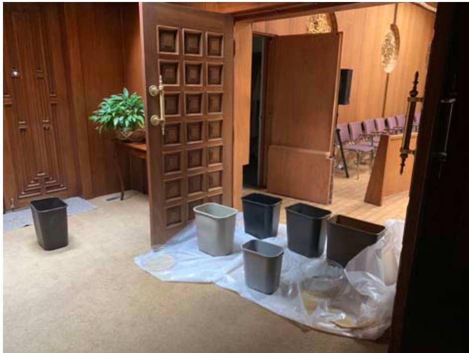
Leaks at Chapel entrance
