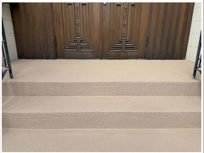
Chancellery front steps (before repair)
