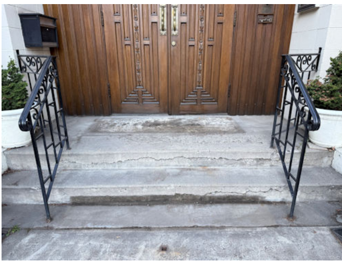
Chancellery front steps (before repair)
