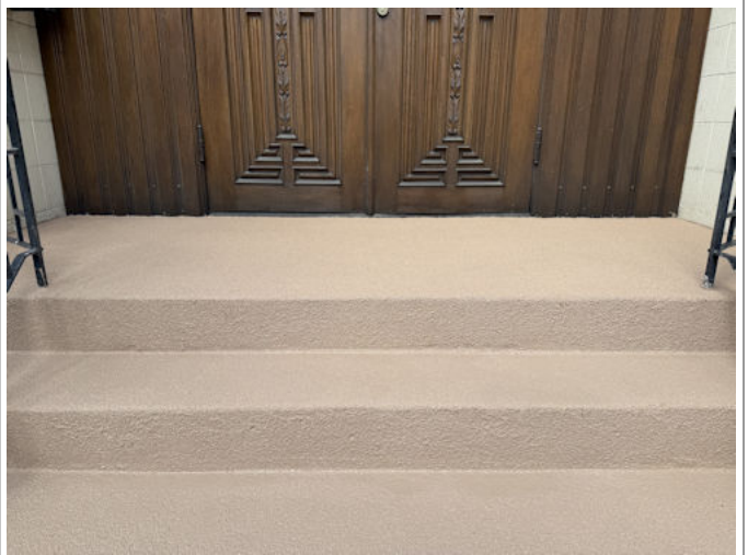
Chancellery front steps (before repair)
