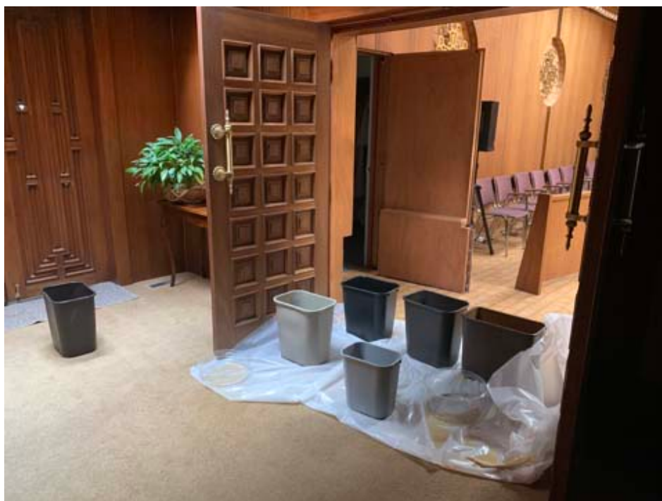
Leaks at Chapel entrance
